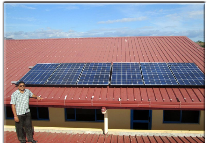
Mr. Ramendra shows the solar panels installed on roof of the B-Block Building.
